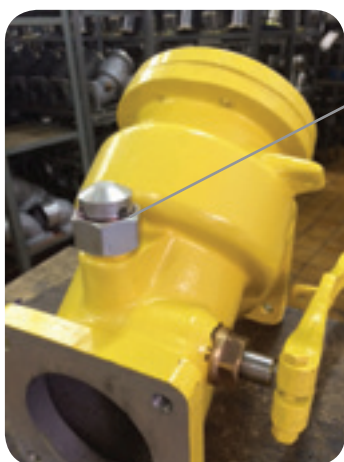
Image 19. Vacuum breaker valve installed.
